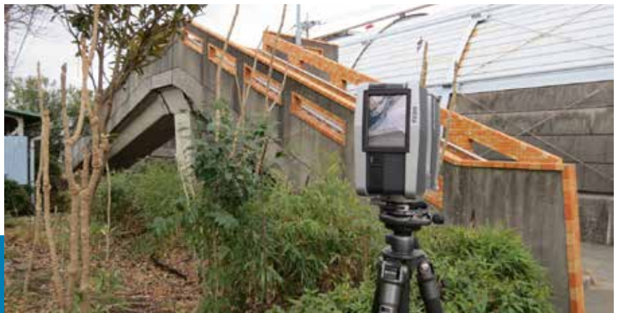
Using the FARO Laser Scanner Focus 3D to scan a pedestrian bridge
